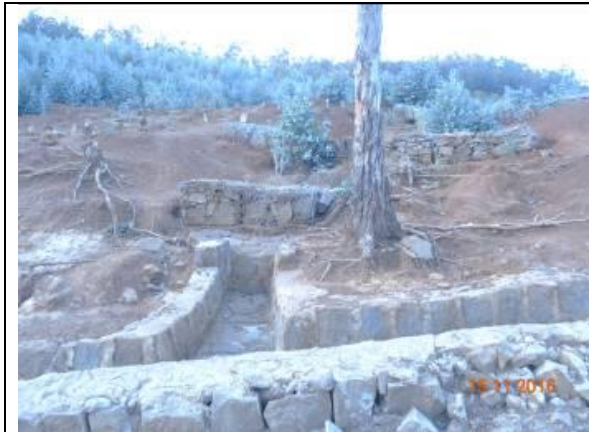
Avert flood, gabion wall and terraces built to prevent soil erosion Yeak 01 Highlands, Addai Ababa City
