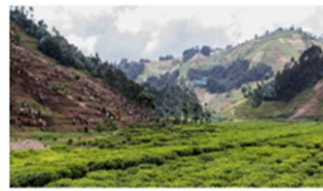
Communities participate in the construction of graded terraces in the steep hillsides in Nyabihu, allowing excess rainwater to run off without damaging the structural integrity of the soil or contributing to erosion. Photo: Rik Moors/One UN Rwanda
