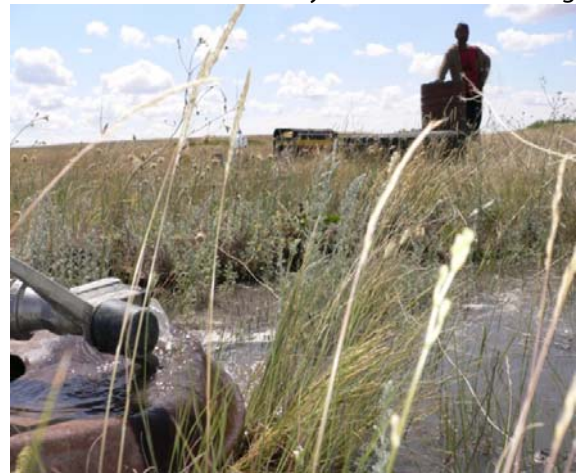
A weir in rehabilitated existing pasturelands and reconstructed water channels for irrigating pasturelands
