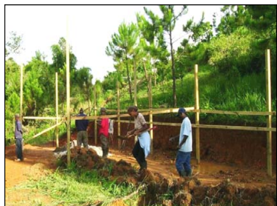
Community members participate in the construction of a greenhouse to be used for organic farming. Photo: JCDT for UNDP CBA
